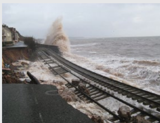
Photo 1.1 Damage to the railway at Dawlish in Devon, the United Kingdom
