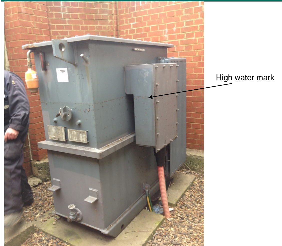
Figure 7.1 - Flooded 11000V transformer at the Port of Dover
