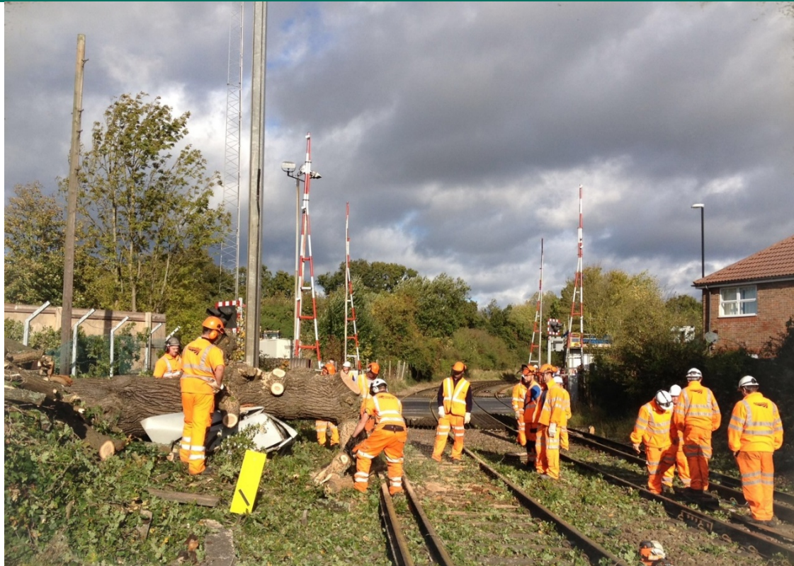
A maintenance team clearing a fallen tree at Keymer, near Brighton.
