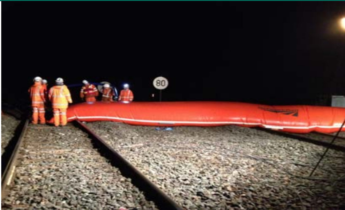
An inflatable temporary dam being put in place to protect infrastructure from flooding.
