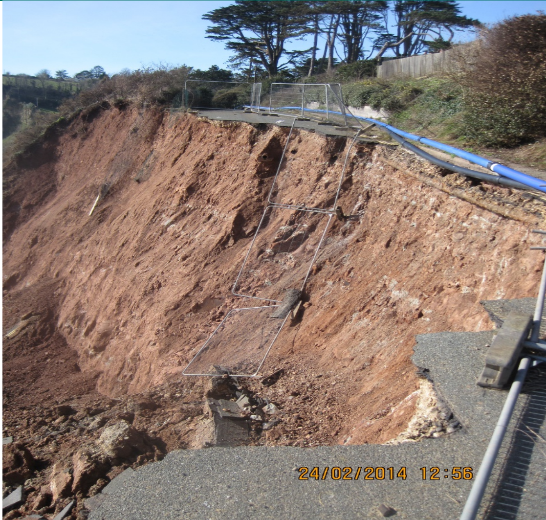
Landslip on local road.
