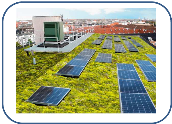
Standard sedum-mos m. solceller
